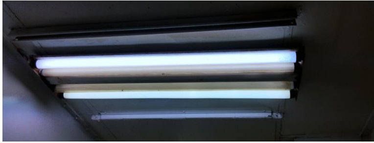
Figure 1: T12 Bulbs within the Facility
