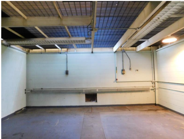
Figure 3: Metal Halide Fixture within the Facility
